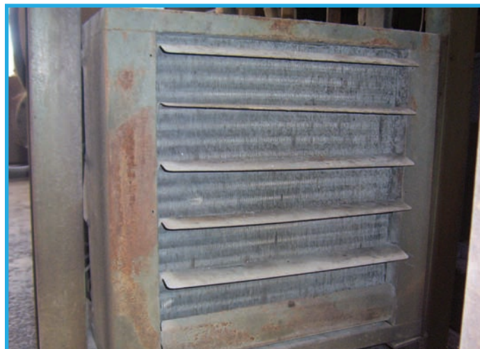
Untreated heat exchanger
